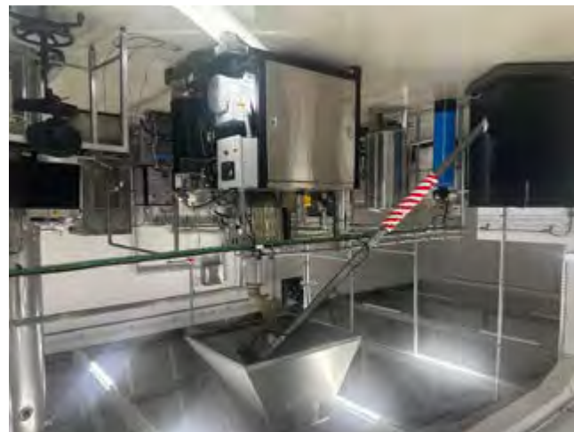
Figure 2. Pilot gasification unit installed on BRIC
