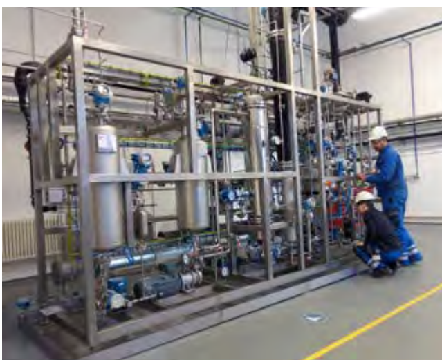
Figure 1. Newly commissioned crude methanol distillation column for tailor-made Maritime Methanol. © Air Liquide (coordinator of the M 2 ARE project).
