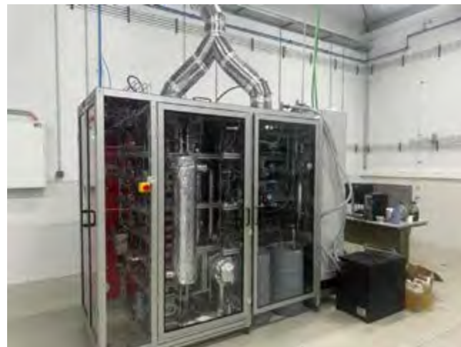
Figure 1. Pilot e-methanol synthesis unit installed on BRIC
